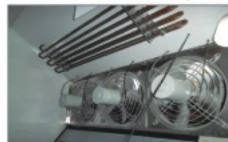
Partition fan, heating and water cooling
