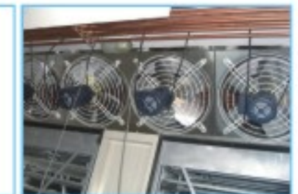
Fan, heating and water cooling system
