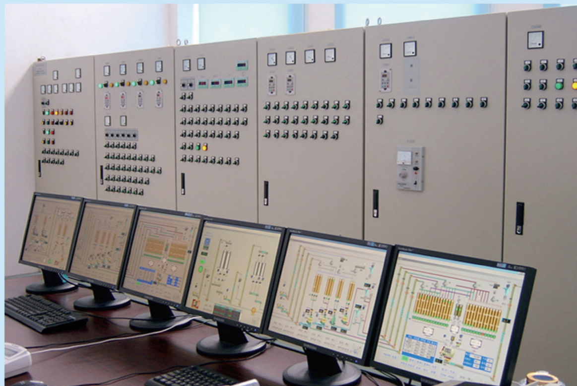
Bus Full Control System
